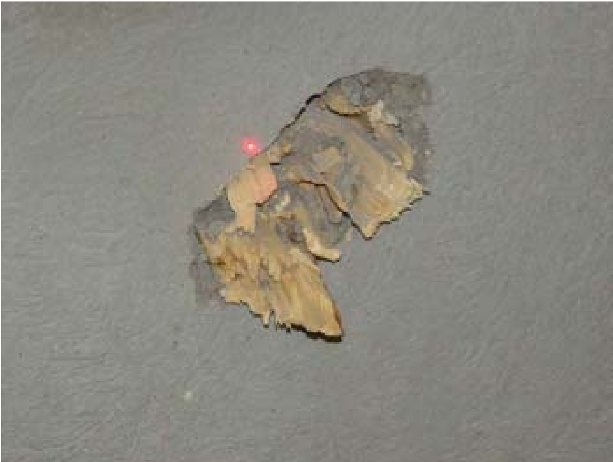
Series 3 Panel Impacted by the Tornado Missile I
