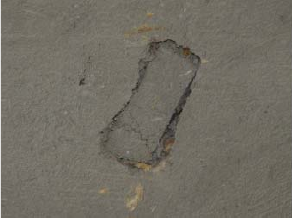
Series 5 Panel Impacted by the Third Tornado Missile
