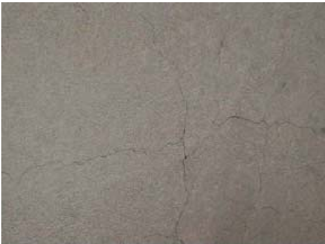
Radial Cracking of Backside of Series 4 Specimen
